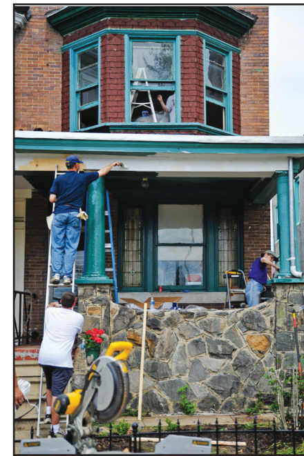
Rebuilding Together Baltimore volunteer team from the Law Offices of Whiteford, Taylor and Preston hard at work making repairs on Alma Lee's house.
